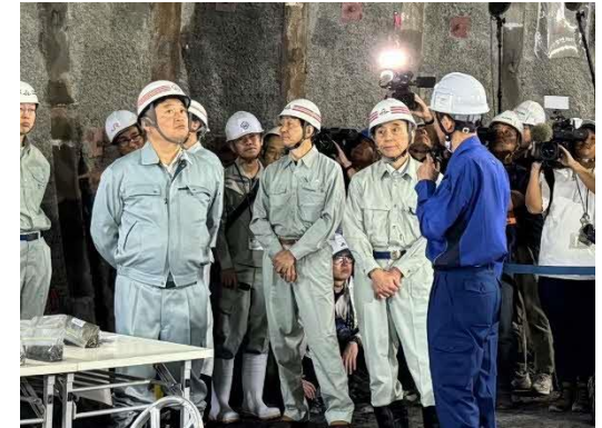
Site visit by the two governors of a high-speed long-range pre-excitation exploratory drilling survey
