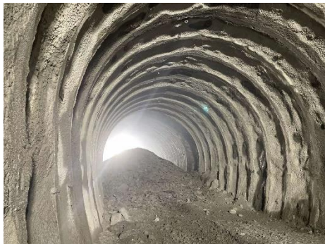
Southern Alps Tunnel (Nagano Section) Pilot tunnel penetration (Nozokiyama Emergency Exit - Kamazawa Emergency Exit)
