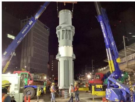
Nagoya Station (Central west section) Construction of a pillar of the underground station building
