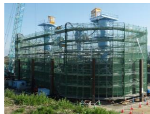
Bridge railing on the Fuefuki River and the Nigori River Pier construction
