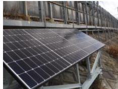
Solar power generation on Shinkansen banking (test installation)
