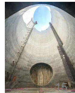
Higashiurigaoka emergency exit
