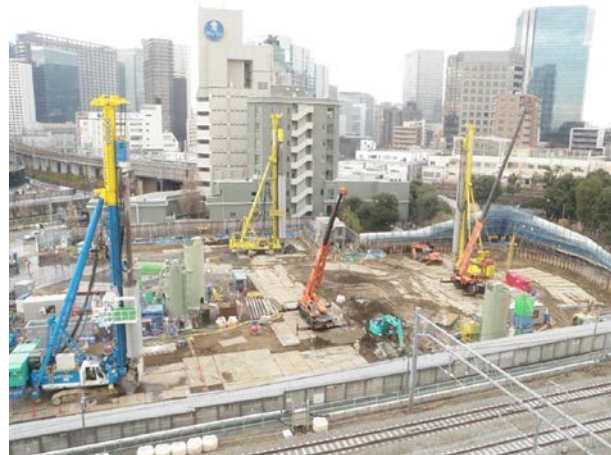
Kita-Shinagawa emergency exit and electrical substation
