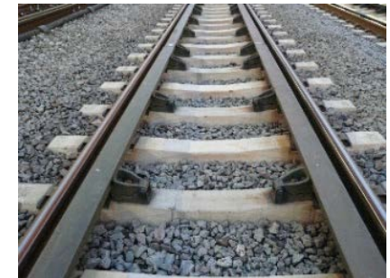
↑ Derailment prevention guards ↑
