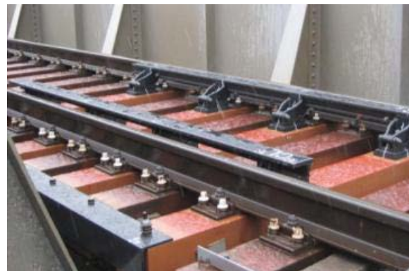
Derailment prevention guards (for non-ballast bridges)
