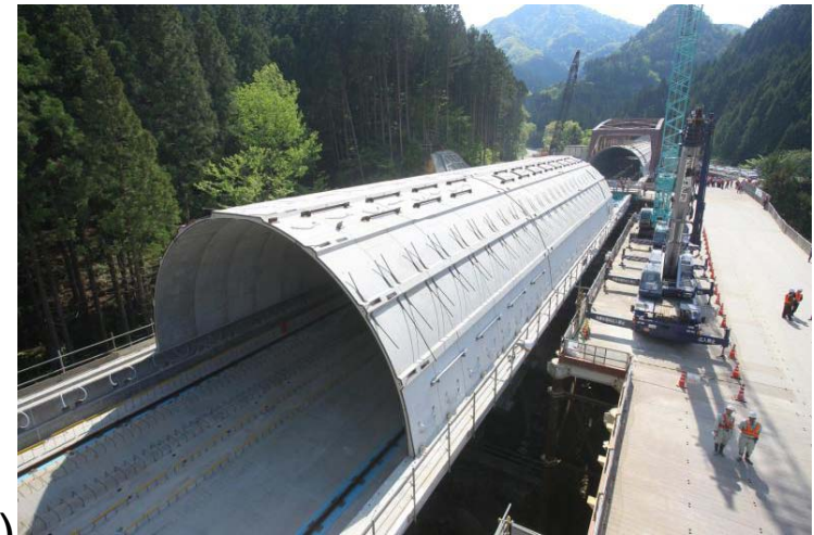
Yamanashi Maglev Test Line Construction Site at the Akiyama region, Uenohara City
