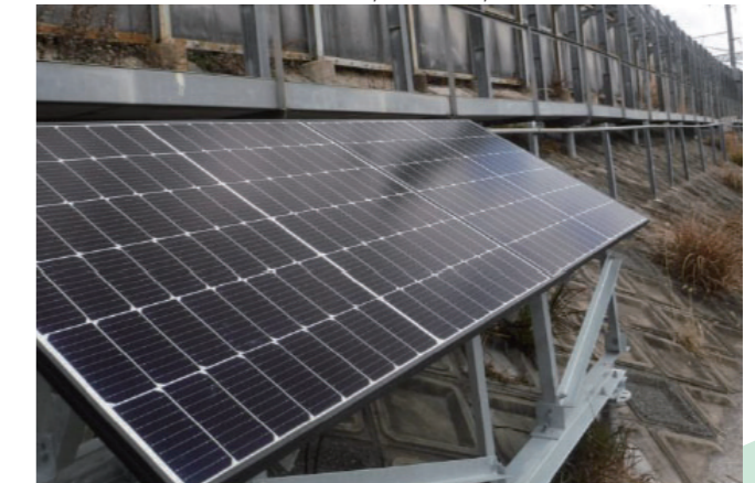
Solar power generation using the Shinkansen trackside slope (trial installation)
